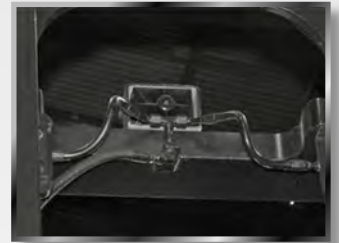
Forward activated alarm
